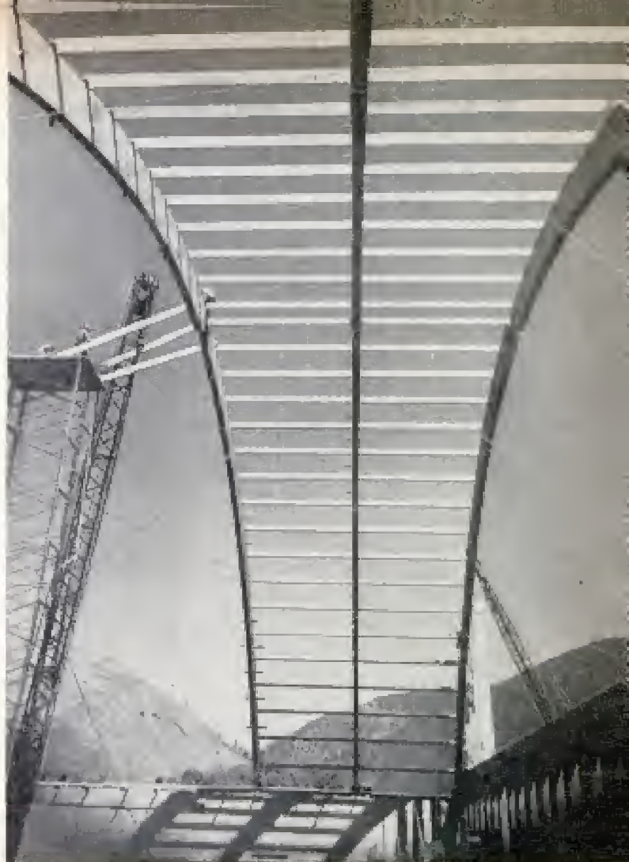
Like a suspension bridge between Montana hills, the roof takes shape. These are said to be the largest such arches ever made
